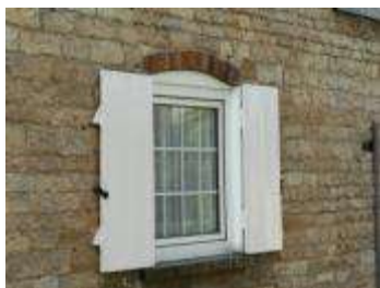
Replacement uPVC windows echo the appearance of the originals, but are not authentic to their functional type. The shutters were once a common feature on estate cottages.
